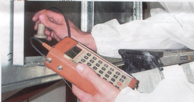
A thorough survey is the best way to assess the state of a ductwork system.
